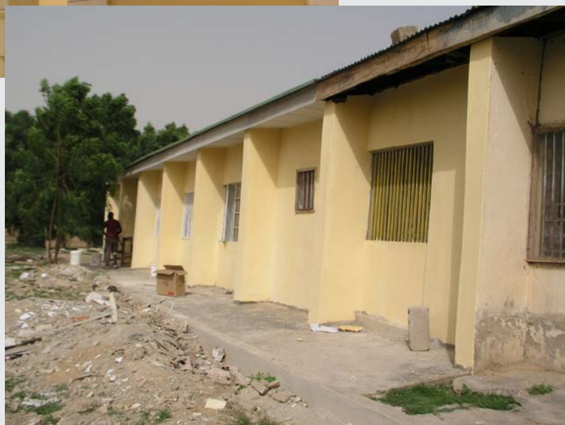
Below: Section of PHC Centre work completed next to an area that work has not yet begun.
